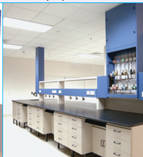
Laboratory Bench with Service Fittings
